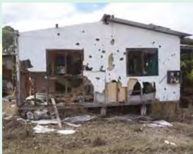
Abandoned asbestos houses on community, can pose a health risk Photo: Ecoteam/Keith Bolton
