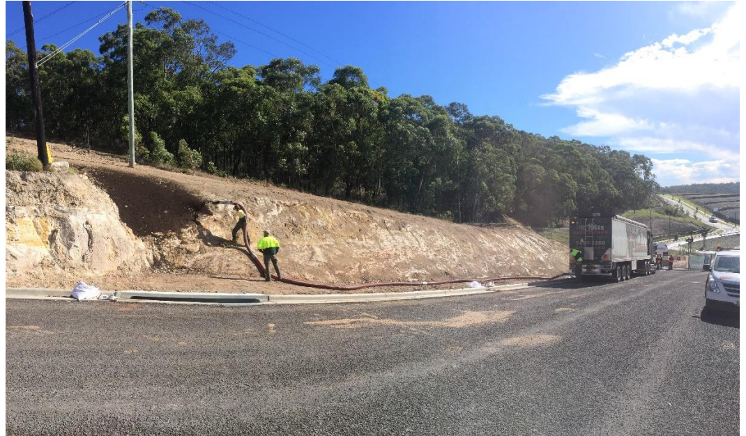
Compost blanket being installed straight onto sandstone batter at the Lake Macquarie site. Photo: The Hills Bark Blower.
