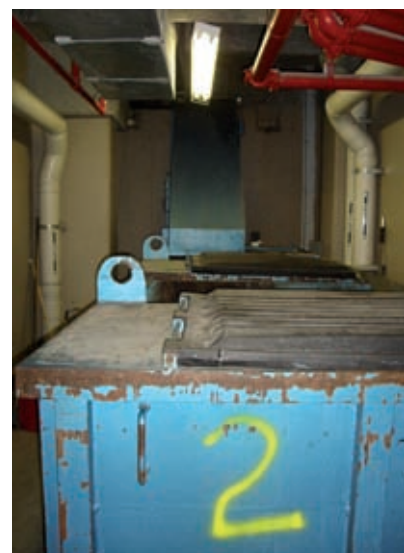
Garbage chute emptying into bulk bins
