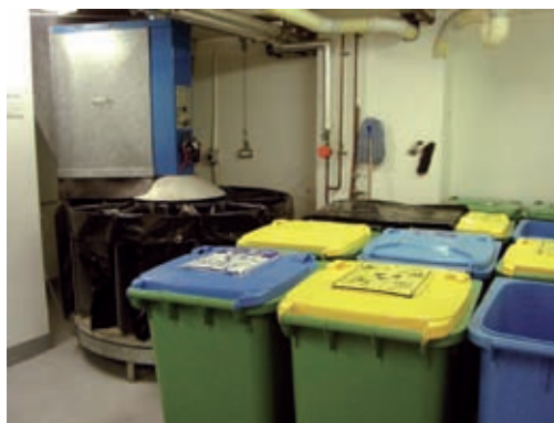
Chute and carousel system and the additional recycling bins for storage of recyclables transferred from the recycling crates located on each level of the building (caretaker access only).
