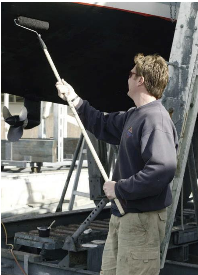
Applying reduced volatile organic compound antifouling paint to a boat hull. Photo: Impress Photography.
