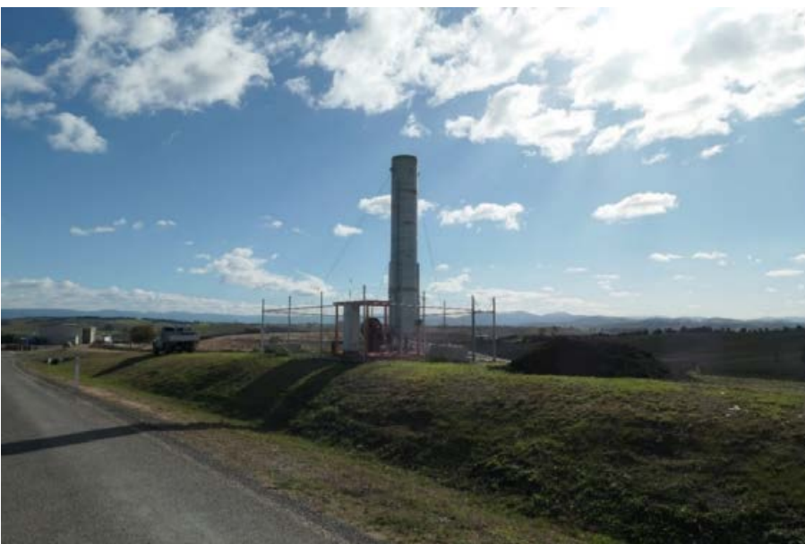
Figure 6 A landfill gas flare. Photo: Karin Schianetz/EPA
