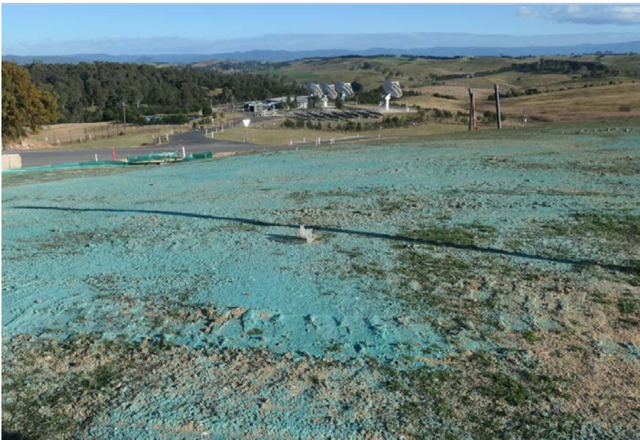
Figure 18 Intermediate soil stabilisation at a waste facility to protect soil from erosion before revegetation. Photo: Karin Schianetz/EPA
