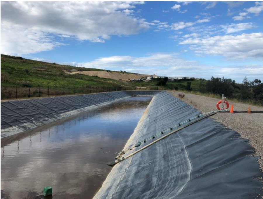
Figure 14 Well-managed leachate ponds with adequate capacity. Photo: Karin Schianetz/EPA
