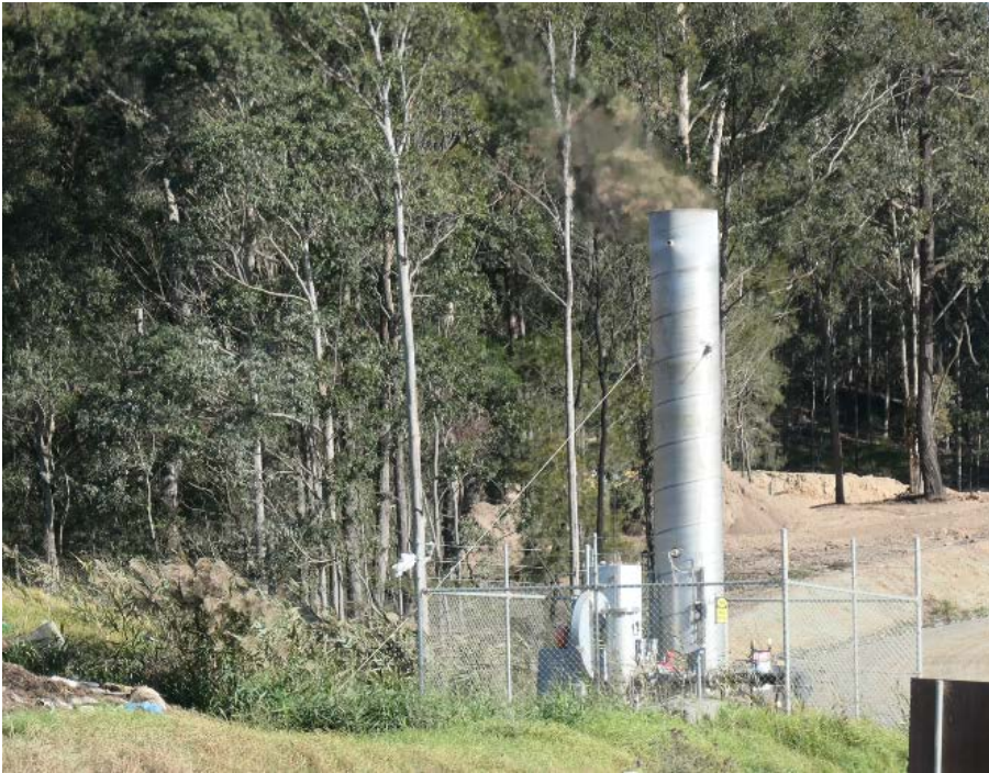
Figure 23 A well-operating landfill gas flare. Photo: Karin Schianetz/EPA
