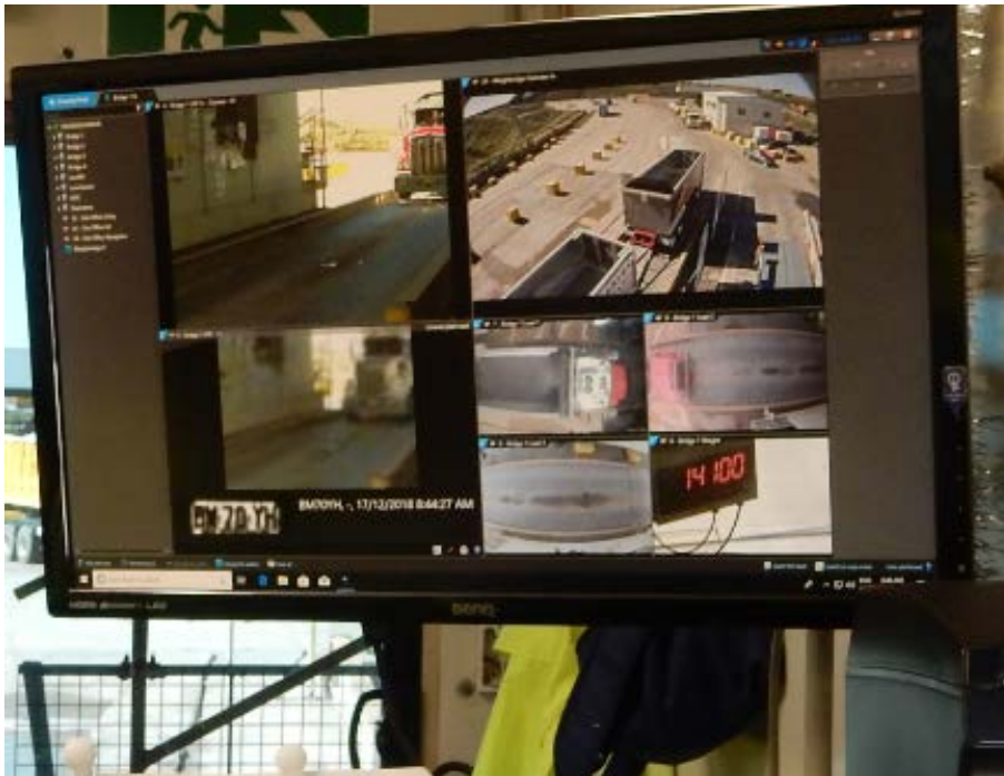
Figure 36 Cameras installed at weighbridge for load inspection. Photo: Karin Schianetz/EPA
