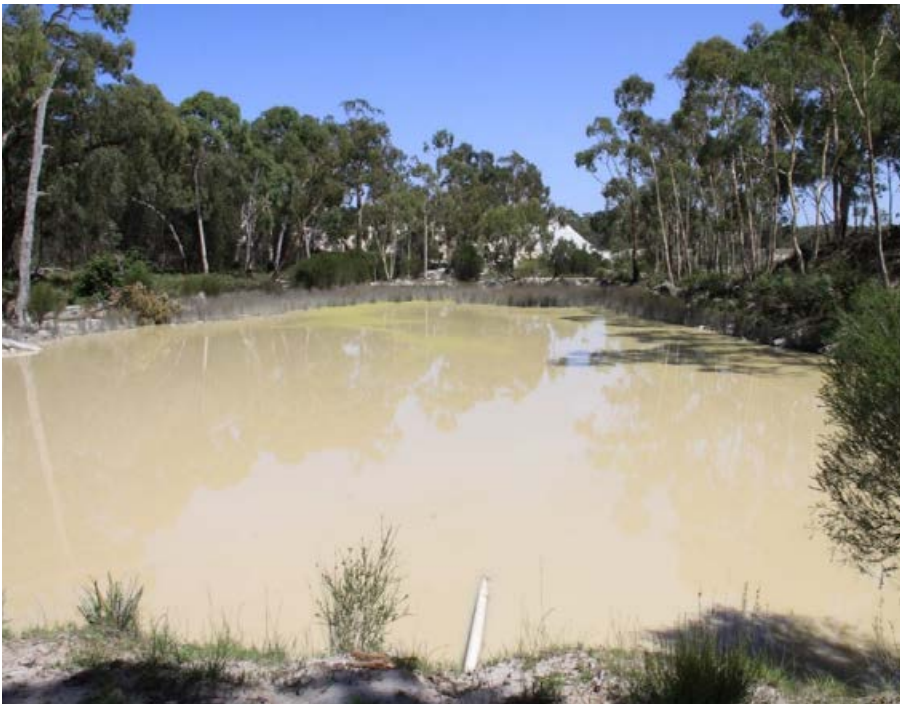
Figure 17 An undersized sediment pond with continuous discharge of sediment-laden water to surface waters. Photo: Karin Schianetz/EPA
