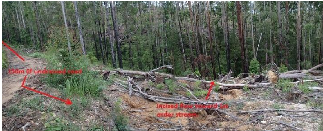
Road drainage (item 22)
