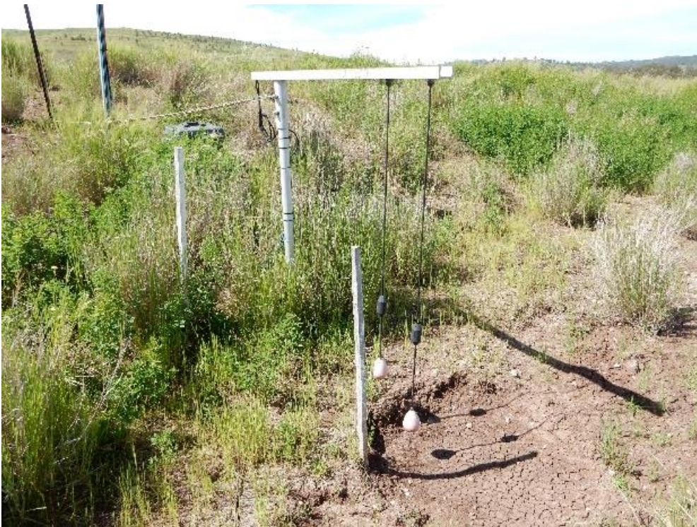
Figure 9: Close up of the float switch system with the high level, and high high level float switches (Photo: E Howard/EPA)
