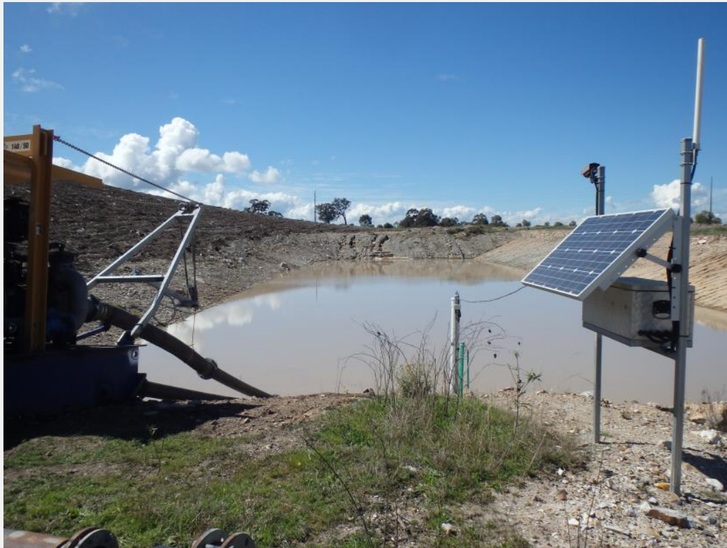
Figure 22: Solar powered automatic water level sensor and webcam installed on a sediment dam (Photo: J Ehmsen/Resources Regulator)
