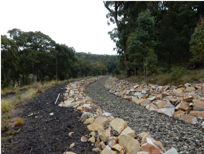
Figure 10: Stormwater diversion drains in place to prevent clean stormwater runoff from entering the tailings and sedimentation dams on site (Photo: M Hatzakis/EPA)
