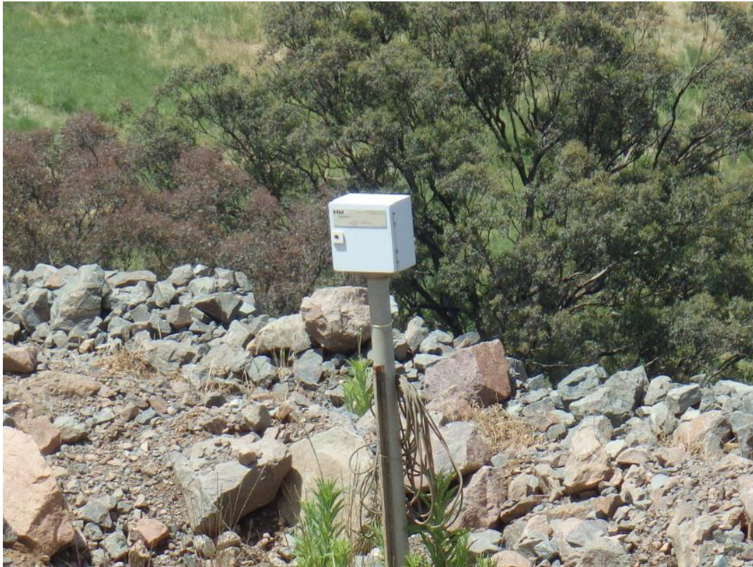
Figure 19: Example of an automatic monitoring piezometer installed on a dam wall (Photo: J Ehmsen/Resources Regulator)
