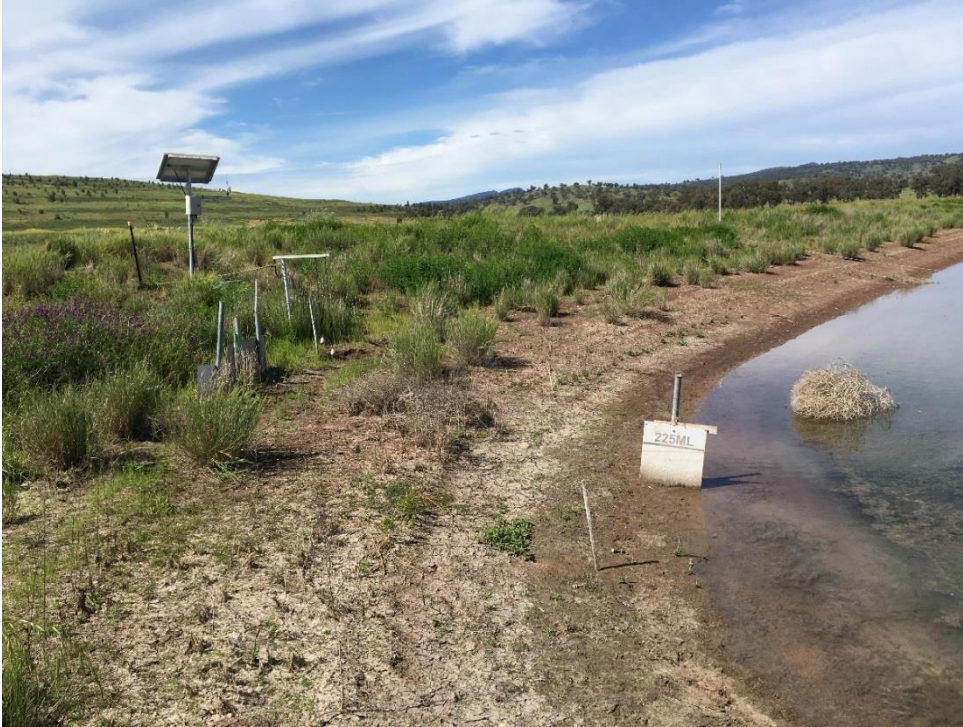
Figure 8: High and high high level float switch system used to monitor water levels in a dam. The system sends an SMS alarm to the operator/s and management when the maximum operational storage level is reached (high level) or when the water level reaches the spillway level (high high level). The information is telemetered using an independent solar power source (Photo: E Howard/EPA)
