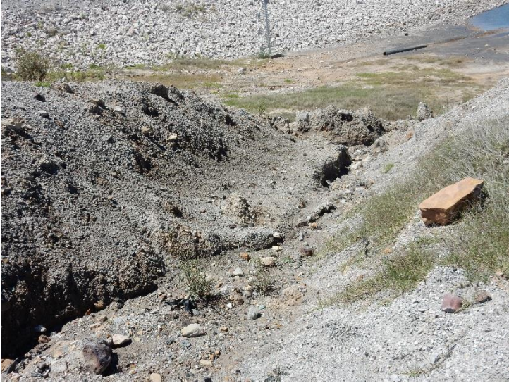
Figure 15: Scouring in emergency spillway (Photo: C Caselia/EPA)
