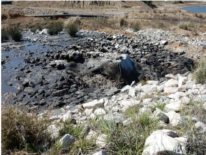
Figure 16: Spillway not properly maintained
