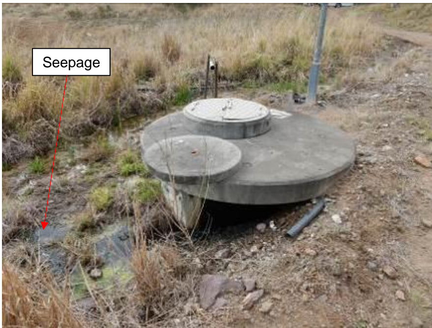
Figure 13: Seepage collection system not being operated properly; seepage was pooling outside the sump and likely to flow to a clean diversion dam (Photo: L Silk/EPA)
