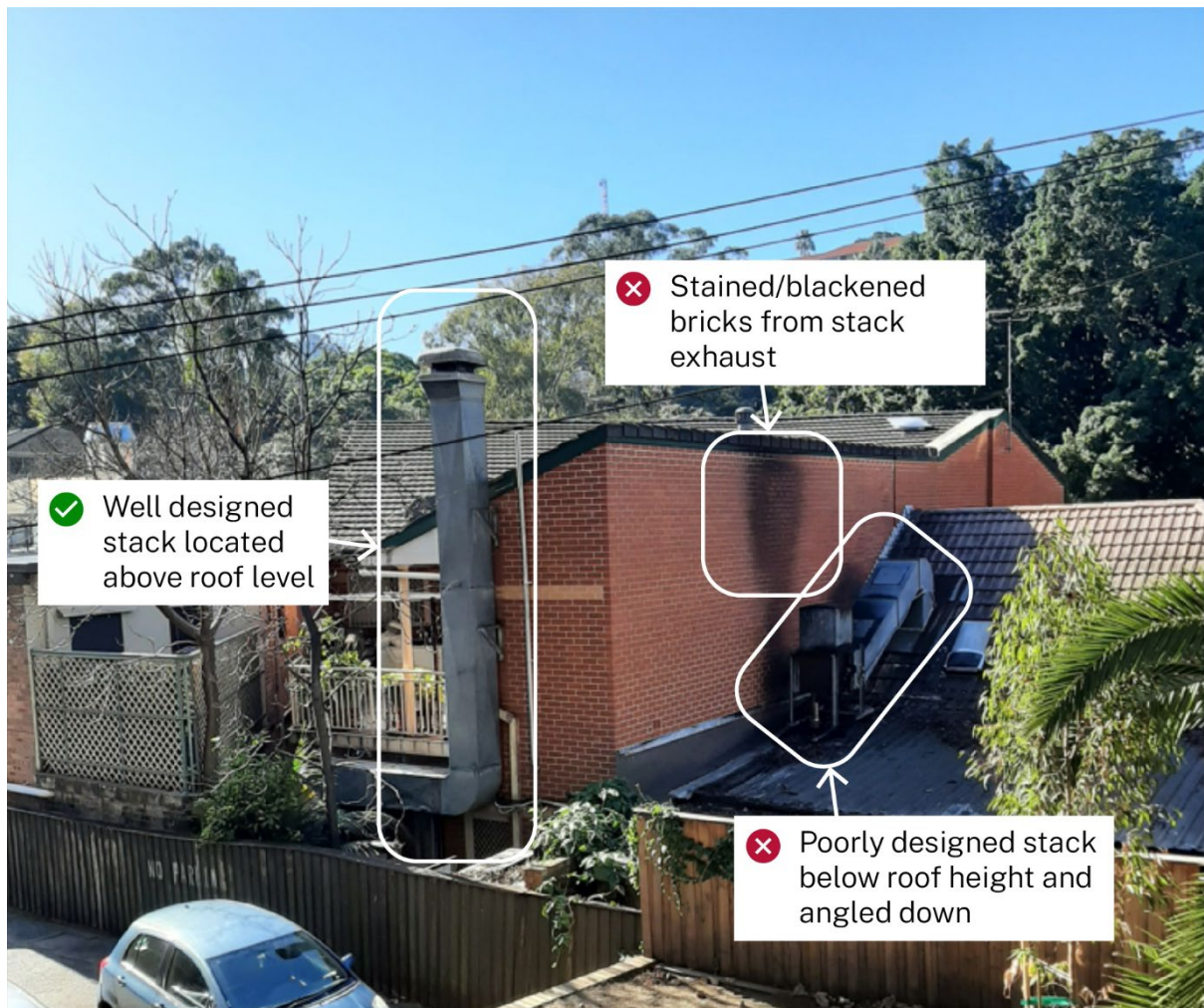
Figure 5 Two stacks, one well designed and one poorly designed and located
