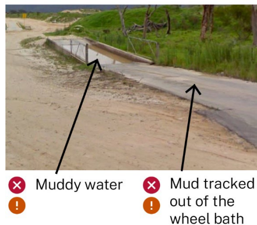
Figure 6 Wheel washing set-up with reduced effectiveness due to muddy water Source: Jane Barnett/Zephyr Environmental
