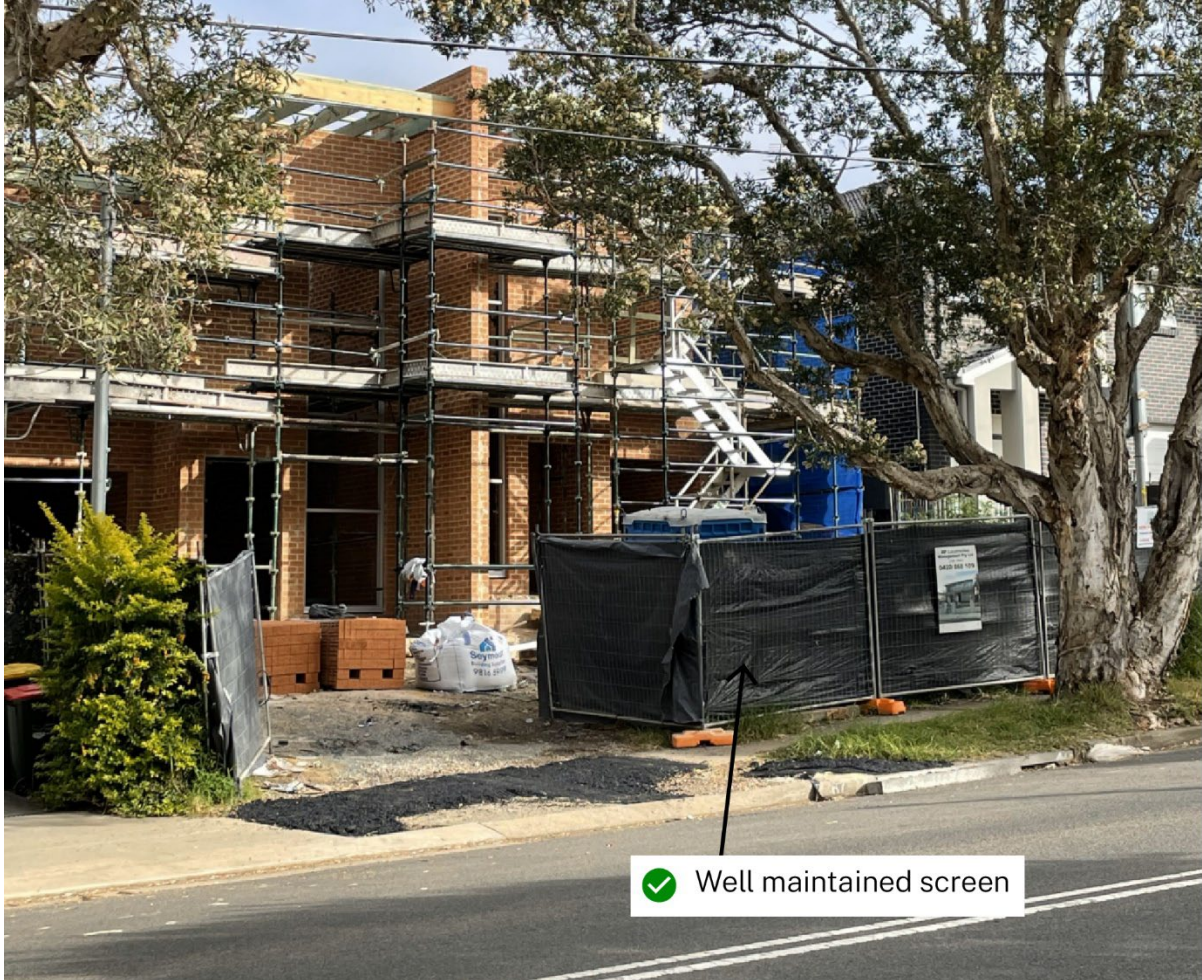
Figure 2 Well-maintained dust screen Source: Jane Barnett/Zephyr Environmental
