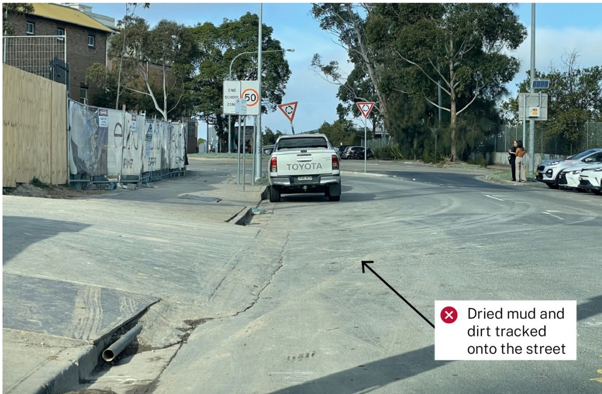
Figure 12 Track-out of dust and dirt from a construction site onto the road Source: Jane Barnett/Zephyr Environmental
