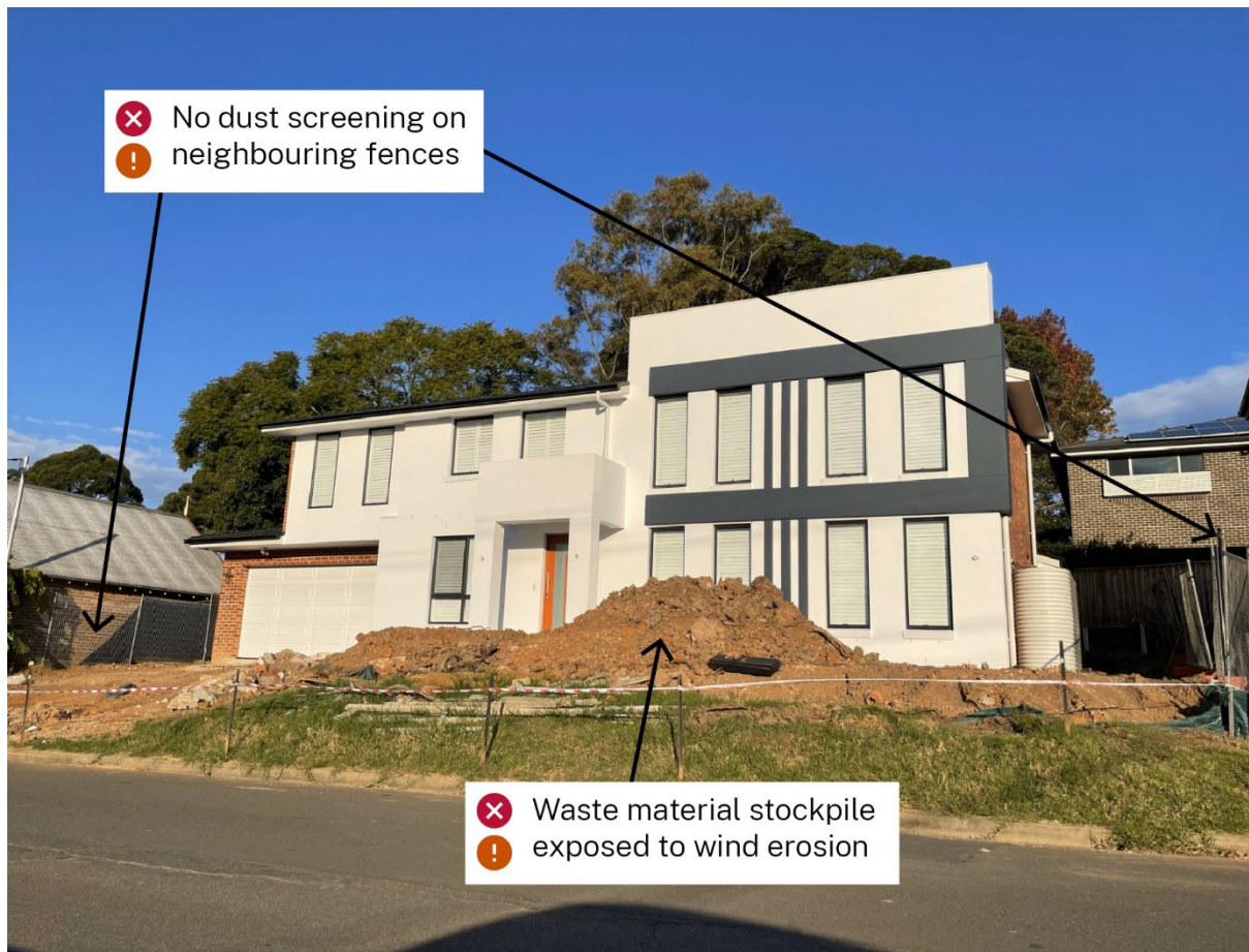
Figure 6 Uncovered building waste and lack of dust screening Source: Jane Barnett/Zephyr Environmental
