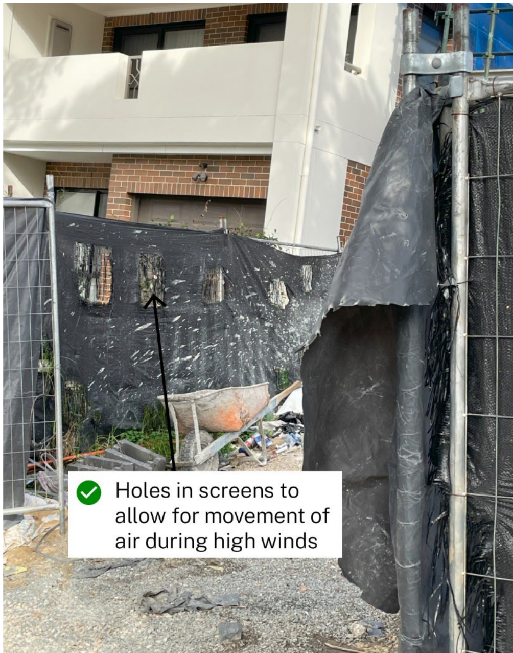
Figure 3 Well-designed dust screen Source: Jane Barnett/Zephyr Environmental
