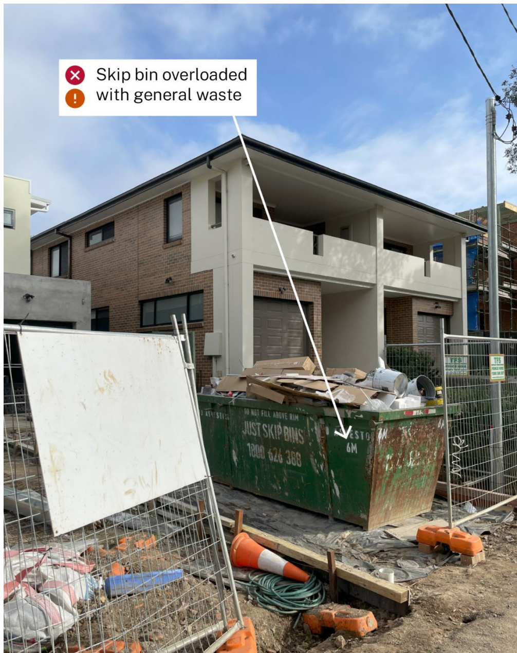
Figure 7 Overloaded skip bin Source: Jane Barnett/Zephyr Environmental
