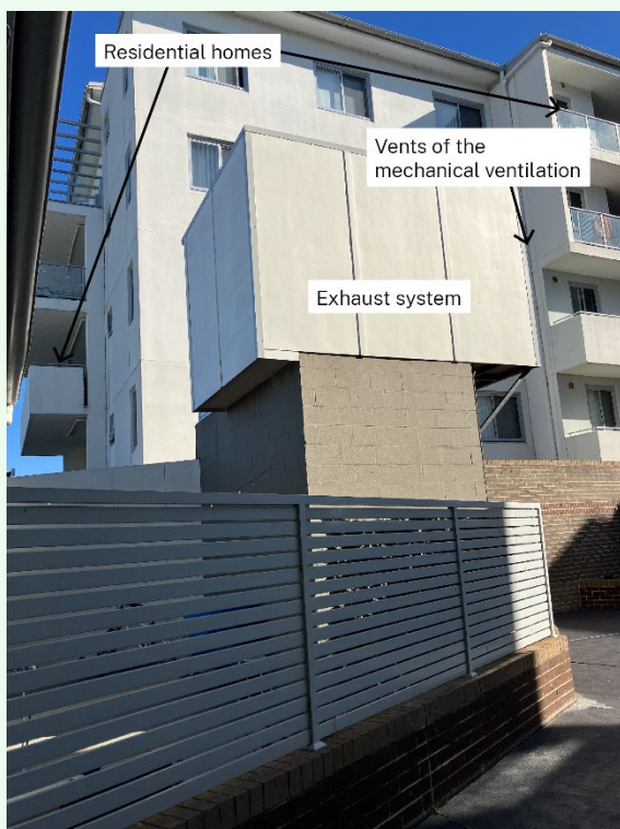
Figure 2 Food outlet exhaust venting near residential properties
